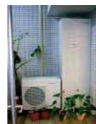
EcoCute Heat Pump Unit (left) and Hot Water Storage Tank
