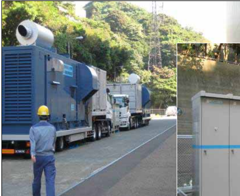
Air-cooled mobile power generators
