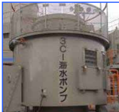
【Deployment of a backup seawater pump motor】 (scheduled to be deployed in March 2012)
